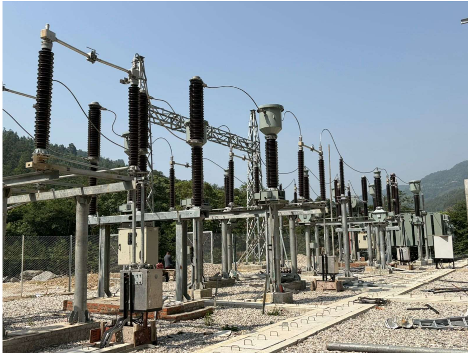
Figure: AP1 Tower at Powerhouse Switchyards
