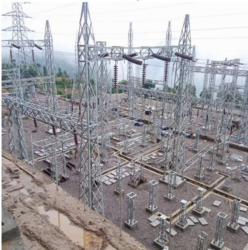
Overall View of LILO
