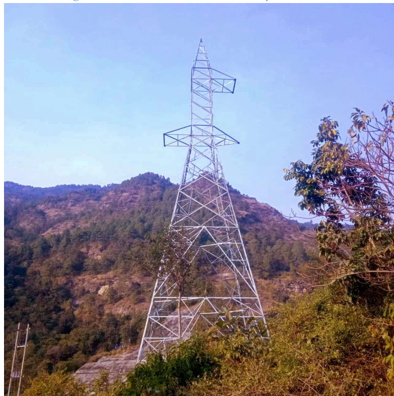
AP2 Tower at Powerhouse Switchyards
