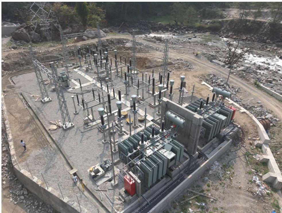
Figure: Power House Switchward
